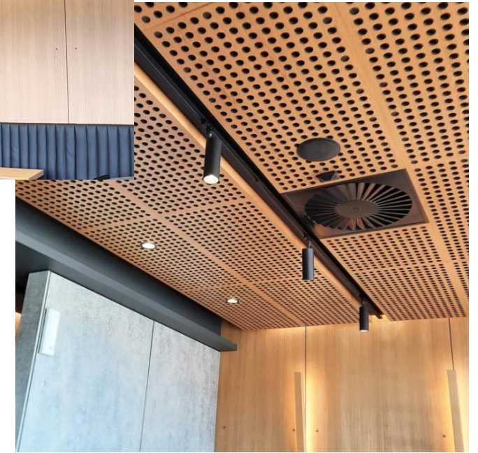
Acoustic Perforated Metal Ceiling + Track Lighting
